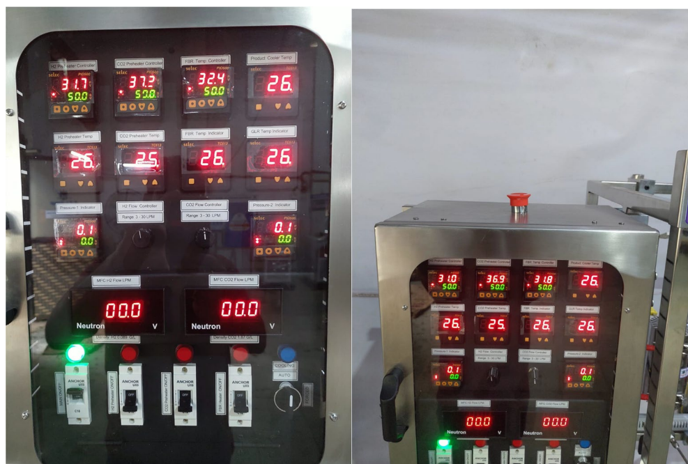
Figure 18: Control Panel of SNG System
