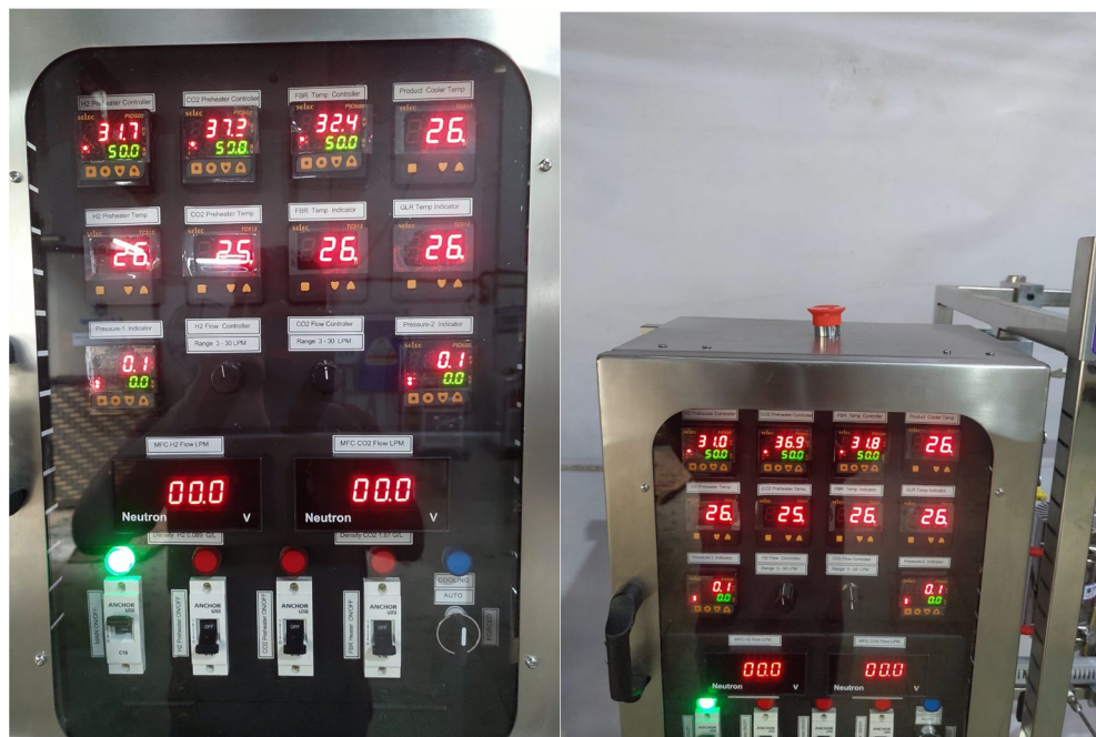
Figure 18: Control Panel of SNG System
